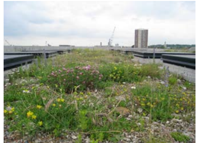
Laban Dance Centre has a Biodiverse roof, designed primarily for biodiversity. The substrate is crushed demolition waste from site, applied on the roof. The substrate varies between 300-700mm and sown with wildflower seeds collected from surrounding brown-field sites.
